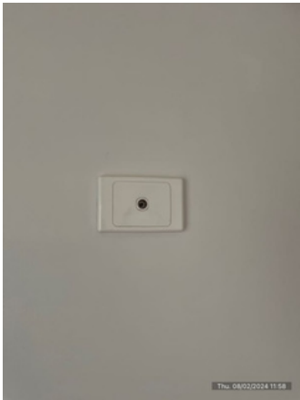
Lounge Room: Lights/power points (photo 2 of 5)
