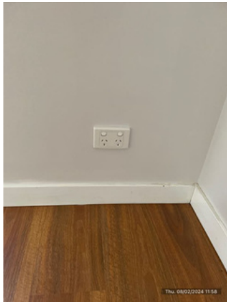
Lounge Room: Lights/power points (photo 3 of 5)
